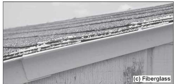
Figure 2. — Side view of installed shingles: (a) western redcedar (WRC), (b) wood-thermoplastic composite (WTPC), and (c) fiberglass.
